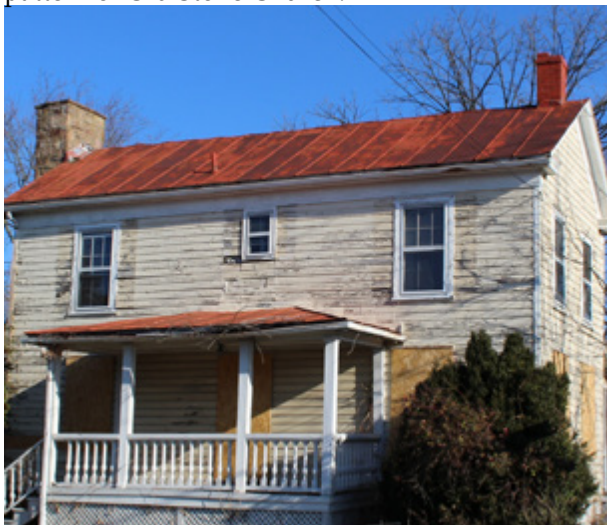
Standing seam metal roof with stone and brick chimneys and a front porch.
