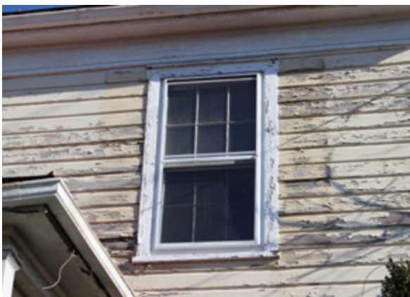
Removing original features, such as shutters (not recommended).
