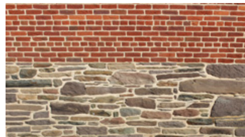
Detail of the stone foundation and brick exterior walls of the Colvin Run Mill.
