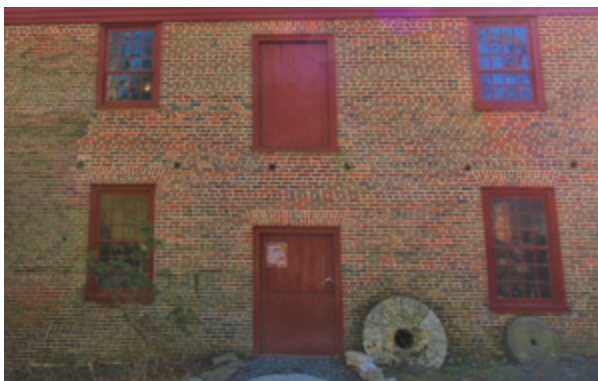
Elevation detail showing typical fenestration (double-hung sash windows and board and batten doors) of the mill.
