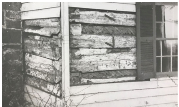
Exposed hand-hewn log structure beneath the weatherboard siding as it appeared during the 1968 move. FCPL, Virginia Room.
