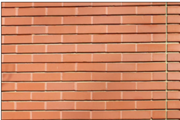
Consistently colored and sized modern pressed brick at the Pope-Leighy House in the Woodlawn HOD.
