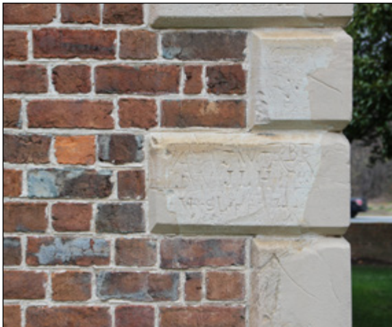
Quoining detailing at the corners of the Pohick Church in the Pohick Church HOD.
