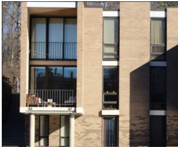
Sliding glass doors with fixed and awning windows in the Lake Anne HOD.
