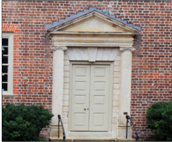
Double-leaf paneled wood door framed by engaged columns and topped with a pediment at Pohick Church.
