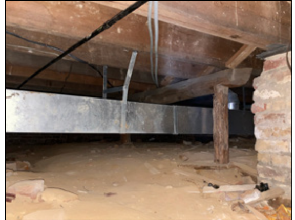
Ductwork installed in crawl space to minimize alteration of historic fabric.
