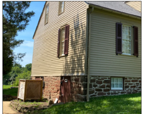
Equipment located on secondary elevation with screening.
