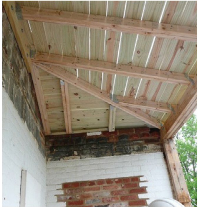
New roof framing of the south porch in 2011 during the restoration. FCPA.
