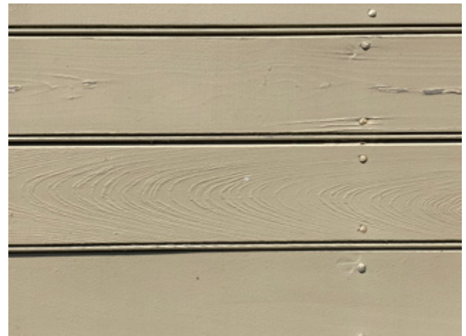
Detail of beaded weatherboard siding featured on the main house, kitchen, office, and smokehouse.
