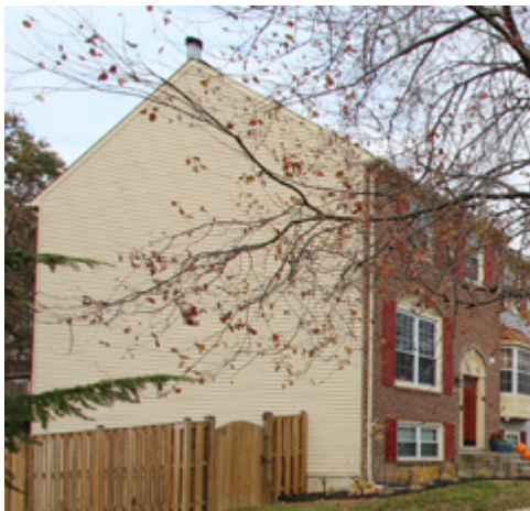
Large expanses of blank walls visible from public streets or sidewalks (not recommended)
