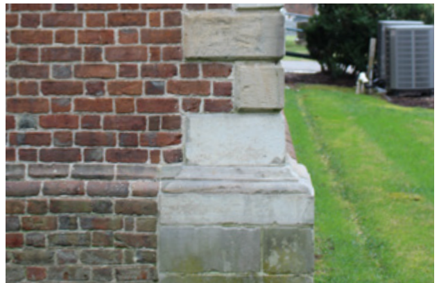
Detail of the stone quoins and brick water table on the exterior.
