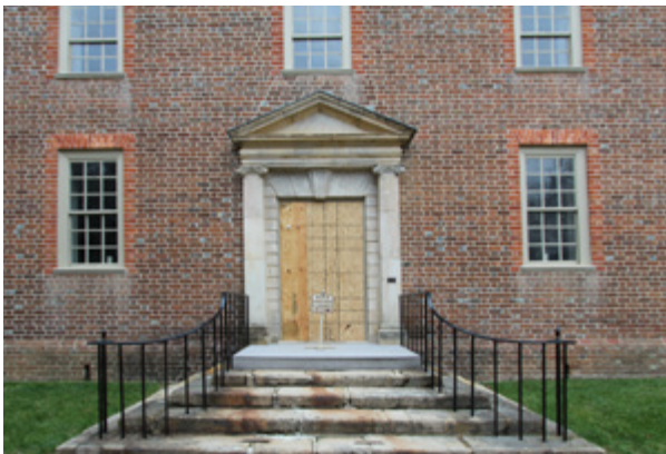
Elevation detail showing the stone steps, main entrance with stone surround, and windows.
